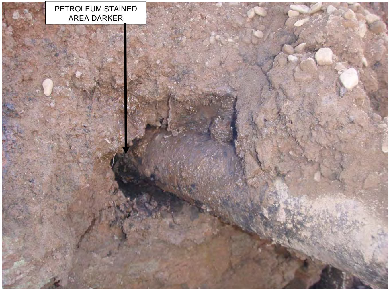
Photo 3-9 This is a photo underneath one of the IOL 4 inch underground gasoline transfer lines showing petroleum product and staining. Location shown in previous photos. Photos 3- 6 and 3-7 shows relative location of pipe with the IOL buildings apparent and Town well noted "for " reference on photos.
