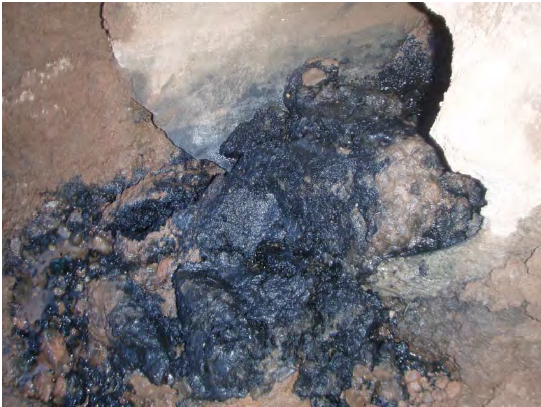
Photo 3-8 Close up shot of petroleum staining for conduit having an orientation that indicates the pipe to be from the IOL bulk plant property. Photos 3-6 and 3-7 shows relative location of pipe with the IOL buildings apparent and Town well noted “for “ reference on photos.
