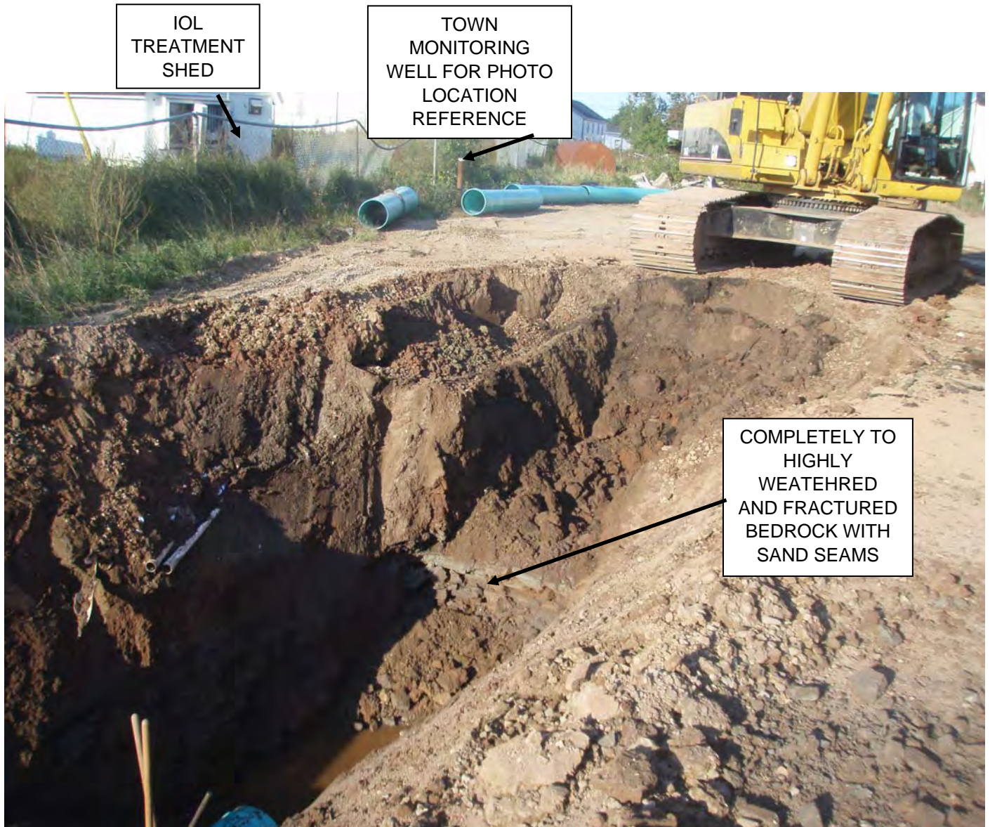
Photo 3-5 Showing highly fractured bedrock.
