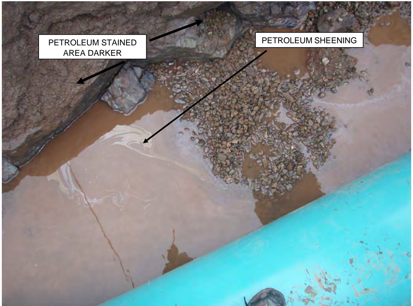
Photo 3-3 showing petroleum sheening in groundwater at TP 3 at back end of MEL property near 14 th St where petroleum sheening was evident in seepage on the wall of the excavation (see Photo 3-2).
