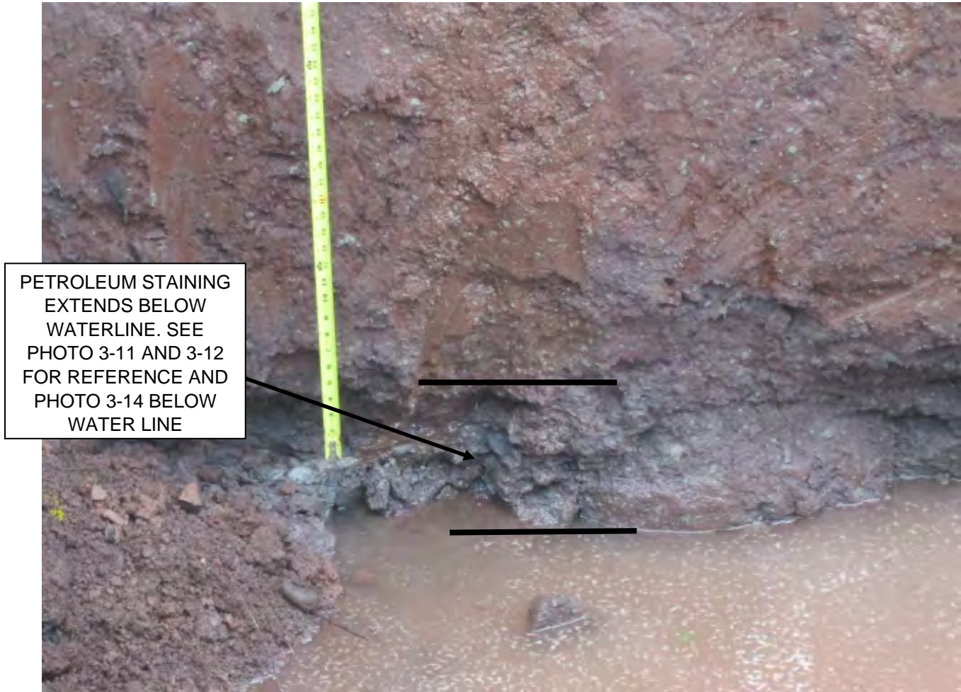
Photo 3-13. Close up of petroleum staining at water line shown in Photo 3-12. See Photos 3-11 and 3-12 for reference location. Underground sewer line at the boundary of IOL bulk plant and 14 th street with new manhole installed. Darker grey area at water line showing petroleum staining. Also see Photos 3-10 and 3-14.
