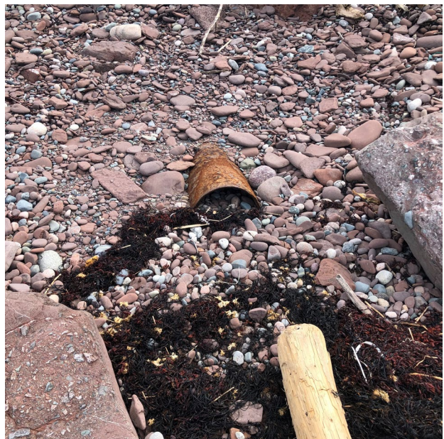
Photo 12 View of Infilled Discharge Pipe from Wetland, Looking North (August 16, 2022)
