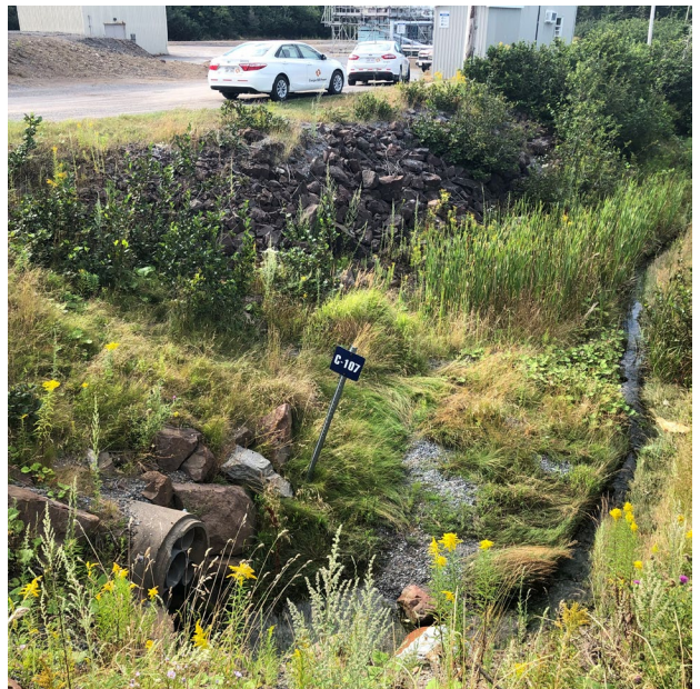
Photo 8 View of Fill Materials on Eastern Bank of Drainage Channel, Looking East (August 16, 2022)
