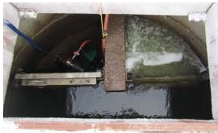
Figure 7: MWWE Toxicity Test Sampling Location - "Rectangular notch" Weir (January 23, 2012)
