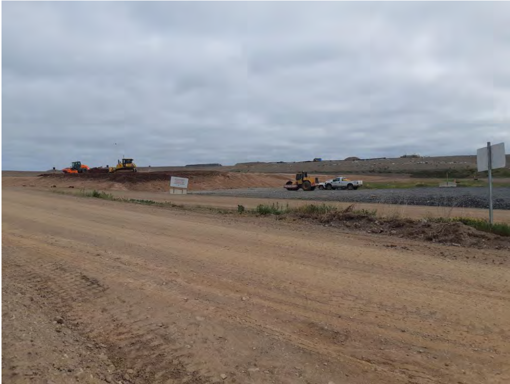
Photo 3: View of the construction of landfill disposal cells in Area E (July 2, 2020).
