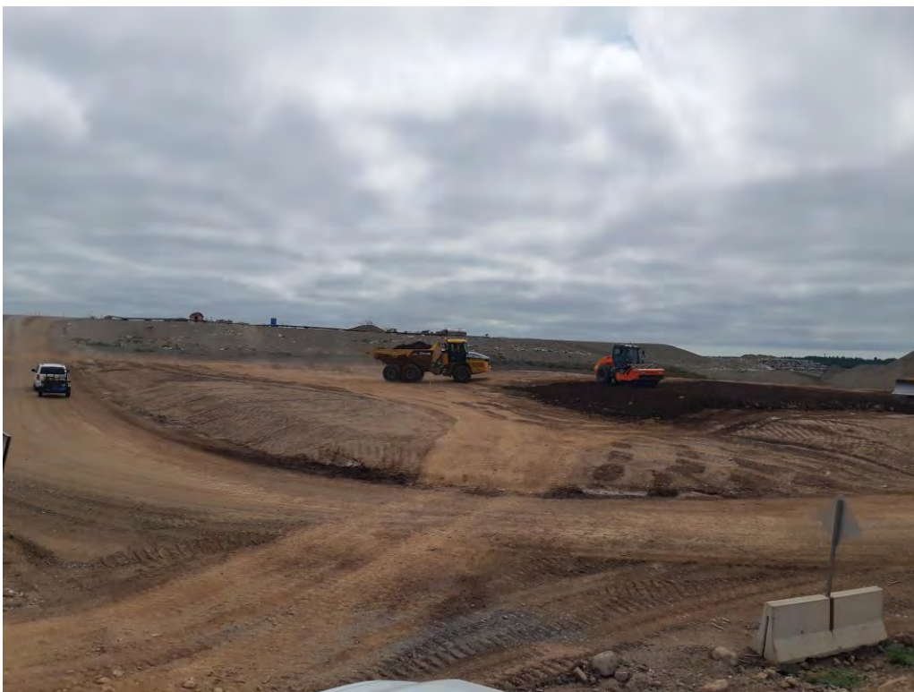
Photo 4: View of the construction of landfill disposal cells in Area E (July 2, 2020).
