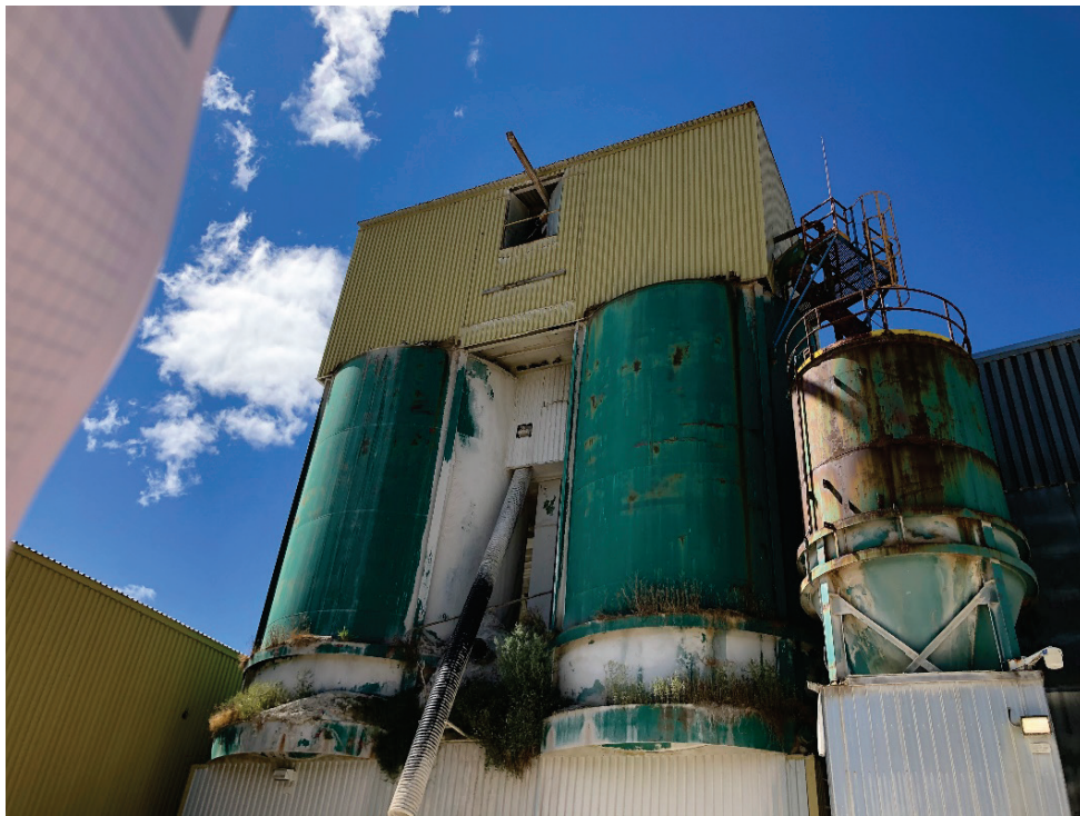
Photo 10 - Photo of stucco storage tanks, looking southwest.
