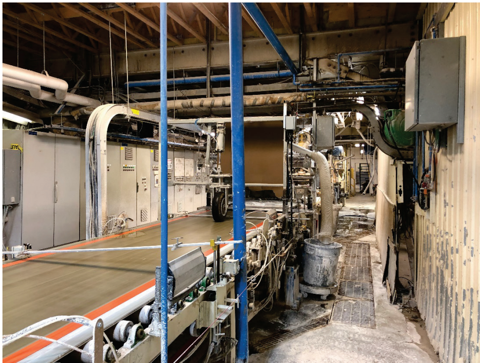
Photo 12 - Photo of wet additives area, leading onto belt #1.
