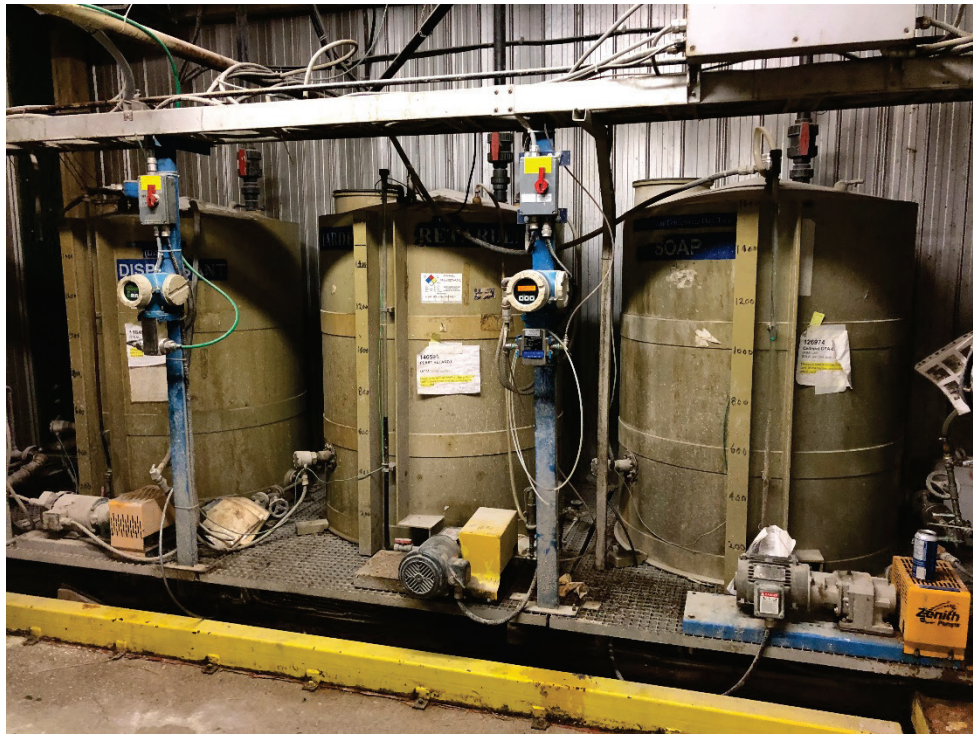
Photo 27 - View of chemical storage tanks in wet additives area.
