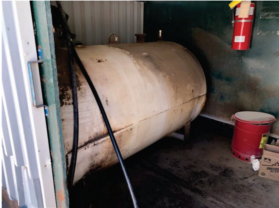
Photo 47 - View of 1,100 L diesel tank located in the Loader Shed.
