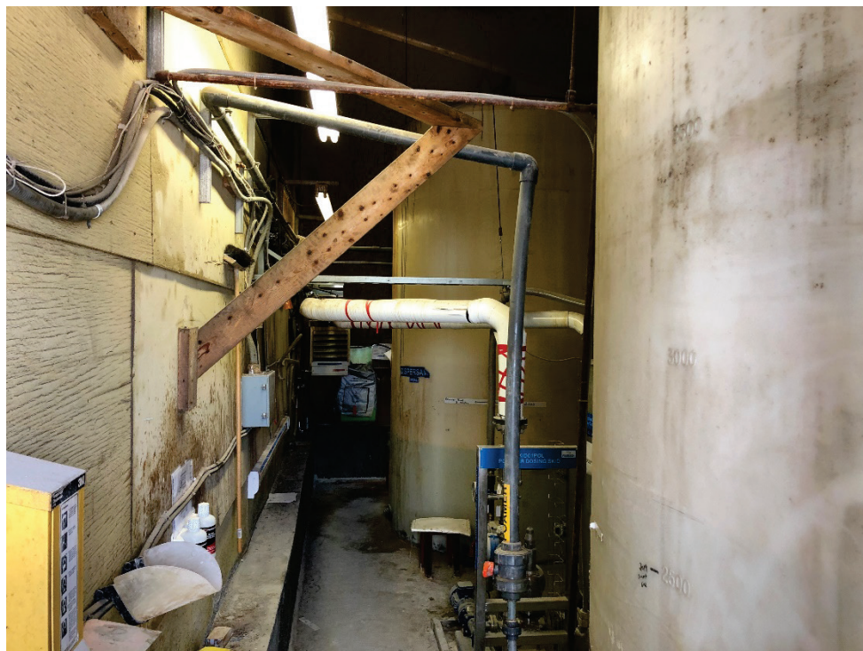
Photo 22 - View of bulk chemical room (Chemical Tanks).
