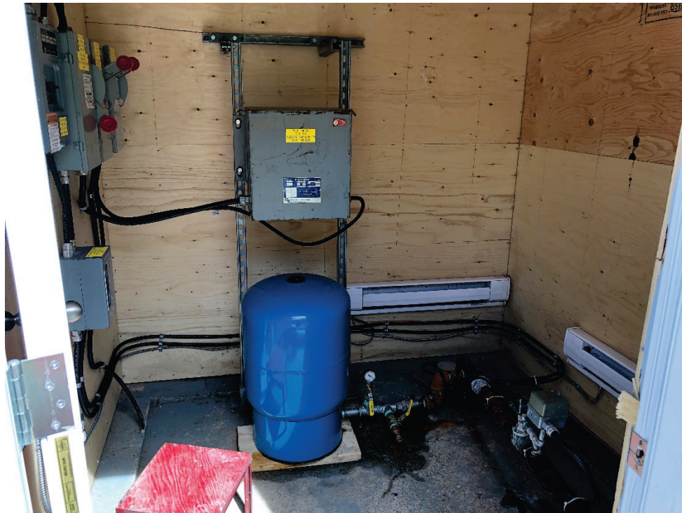
Photo 40 - View of one of the onsite well houses.
