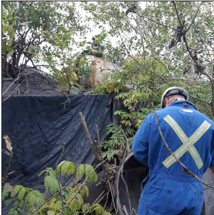
PHOTO 6 - FILTRATE TANK IN DUMP BOX
