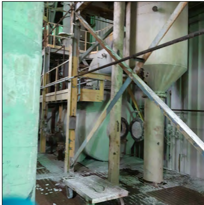
PHOTO 14 - BAROMETRIC CONDENSOR AND EJECTOR SET ON THE 4TH FLOOR OF PAP BUILDING
