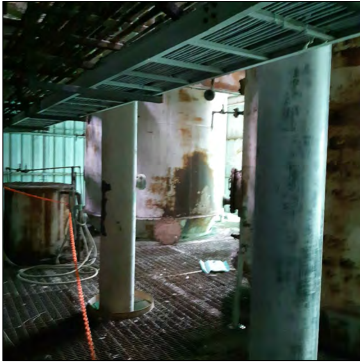
PHOTO 11 - EVAPORATOR TANKS ON THE 3RD FLOOR OF PAP BUILDING
