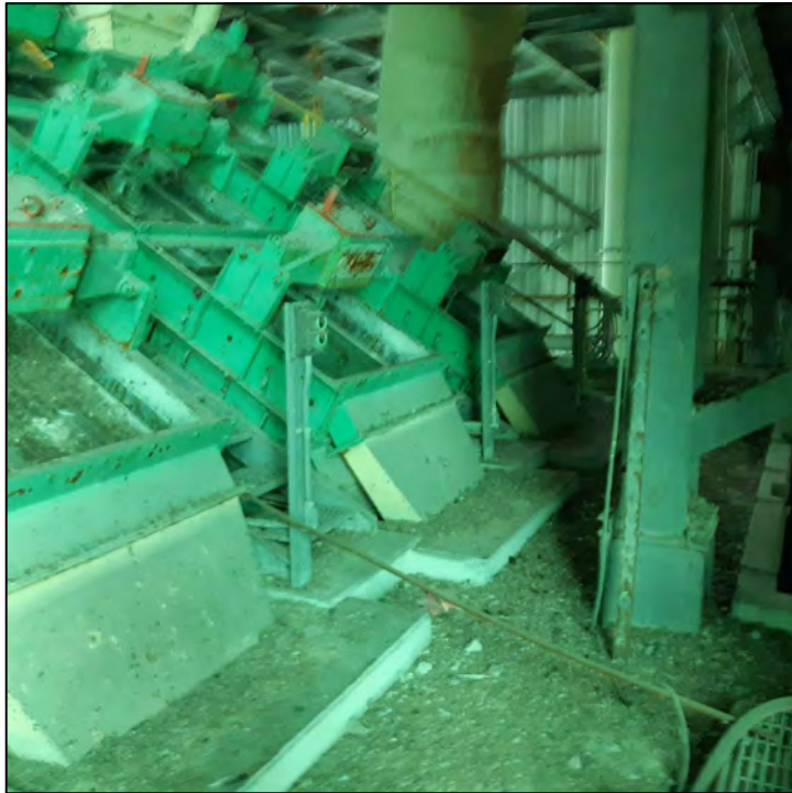
PHOTO 20 - CONVEYORS ON THE 4TH FLOOR OF THE DAP BUILDING
