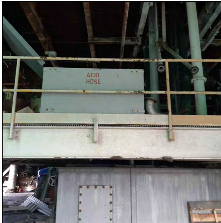
PHOTO 7 - FILTRATE TANK IN PAP BUILDING
