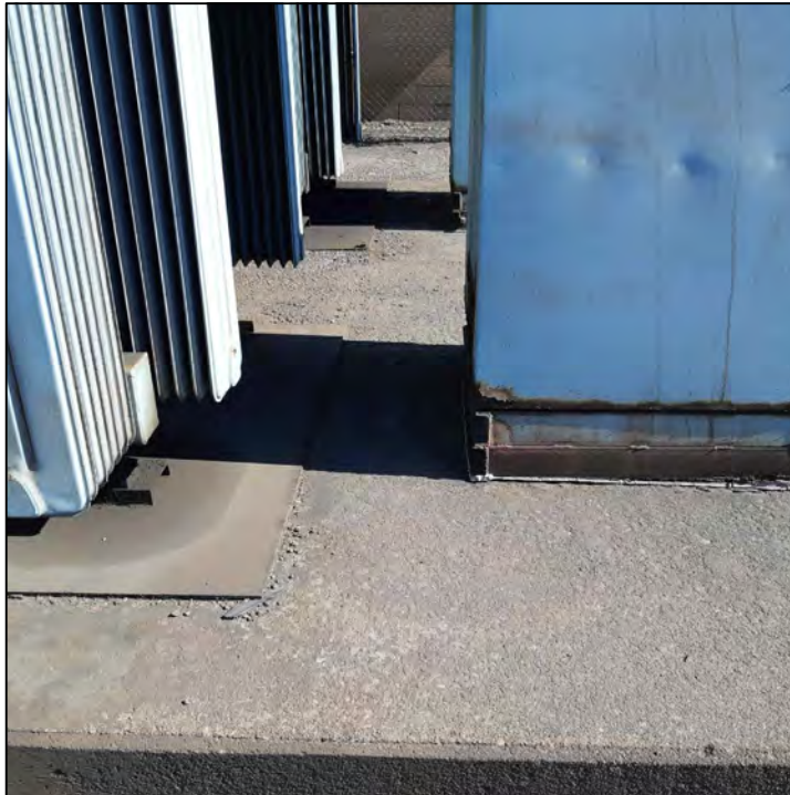
PHOTO 22 - CONCRETE PAD AND TRANSFORMERS OUTSIDE OF THE DAP BUILDING
