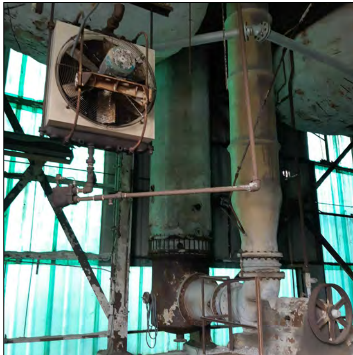
PHOTO 8 - EVAPORATOR PIPING ON MAIN FLOOR IN PAP BUILDING
