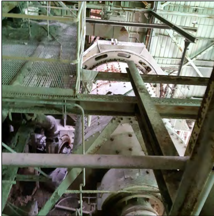
PHOTO 9 - BALL MILL IN PAP BUILDING
