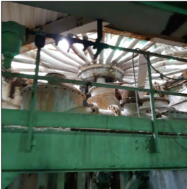
PHOTO 10 - 3RD FLOOR OF THE PAP BUILDING DIRECTLY UNDER FILTER PANS WITH SUSPECTED ELEVATED NORM READINGS
