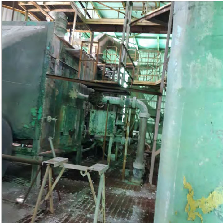
PHOTO 15 - FUME SCRUBBER ON THE 4TH FLOOR OF THE PAP BUILDING
