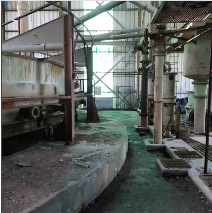
PHOTO 12 - TOP FLOOR OF PAP BUILDING WITH EVAPORATOR TANKS RIGHT AND FILTER PANS LEFT
