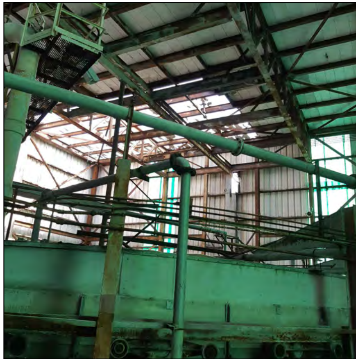
PHOTO 13 - HOUSING FOR PAN FILTERS ON TOP FLOOR OF PAP BUILDING, LOCATION OF 19ACM-4
