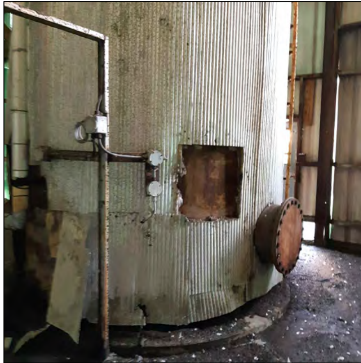
PHOTO 17 - TANK IN NORTHEAST CORNER OF DAP BUILDING ON MAIN FLOOR
