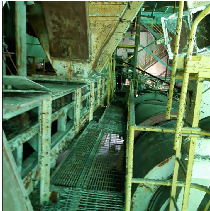
PHOTO 18 - 2ND FLOOR OF THE DAP BUILDING, CONVEYOR ON LEFT AND DRYER ON RIGHT
