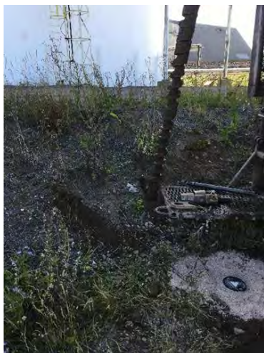
Photo #5: View of the newly constructed monitor well 19GW122 located to the north of the acid tanks.
