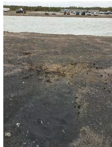
Photo #10: View of the newly constructed soil probe 19SP-19 located north of the cooling recycling pond.
