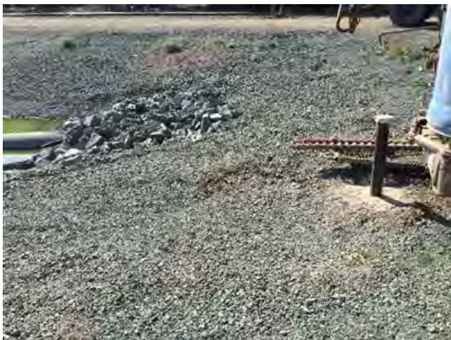
Photo #3: View of the newly constructed monitor well 19GW-118 located adjacent to the acid tank area and the newly constructed bulk pond.
