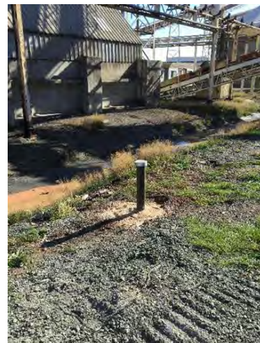
Photo #4: View of the newly constructed monitor well 19GW-120 located within the Material Handling West facility.
