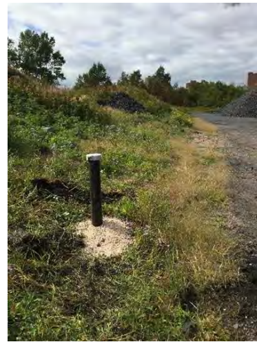
Photo #2: View of the newly constructed monitor well 19GW-114 located adjacent to the Coke Fines.
