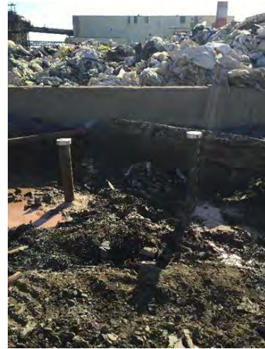
Photo #8: View of the newly constructed monitor wells 19GW133/19GW-134 located to the north of the processed sludge and garbage storage area.
