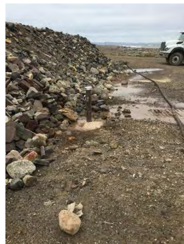
Photo #6: View of the newly constructed monitor well 19GW-126 located to the southeast of the polishing pond.
