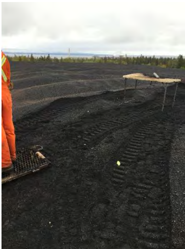
Photo #11: View of the newly constructed soil probe 19SP-26 located on the Slag Pile.
