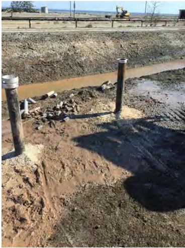
Photo #7: View of the newly constructed monitor wells 19GW127/19GW-128 located to the north of the Back 50.
