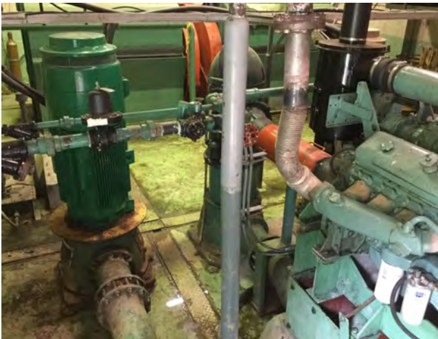
Photo #39: Inside view of the Jacquet River Pumphouse.
