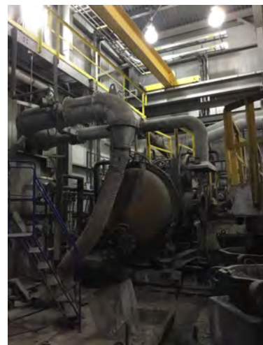
Photo #12: Inside view of Silver Refinery.
