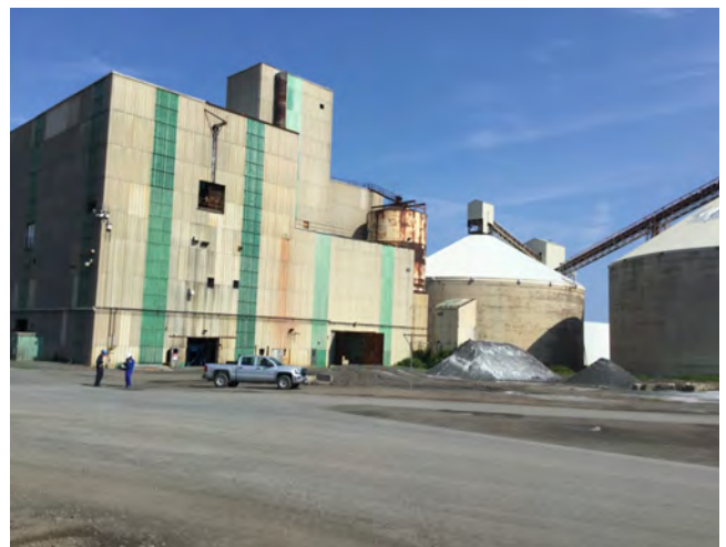
Photo #48: View of the PAP Building with Storage Silos in the background.
