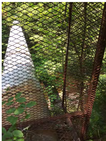
Photo #53: View of freshwater pipeline crossing Belledune River.
