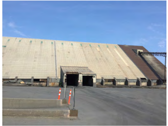
Photo #44: View of the Battery Storage Building.
