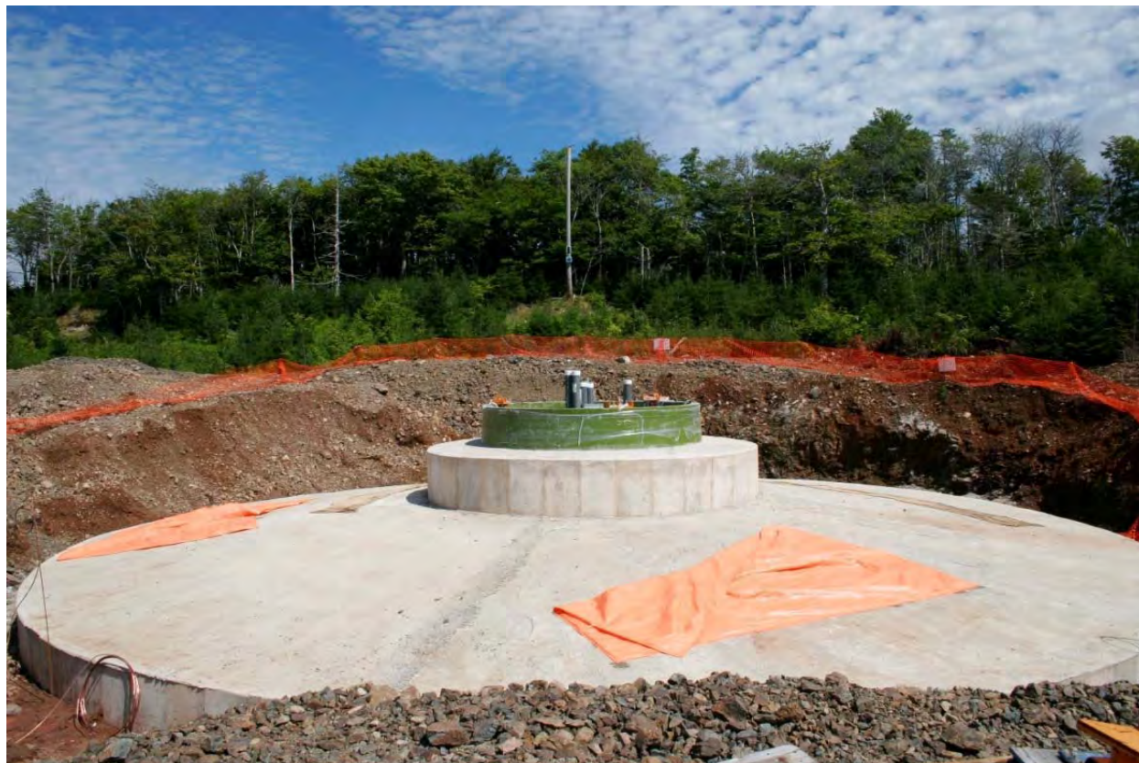
Figure 2-5: Finished concrete foundation for Natural Forces' Fairmont Wind Farm in Nova Scotia.
