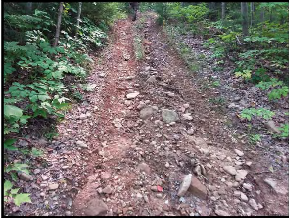
Photo 3: Example of damage from drainage down steep section of Trail I.
