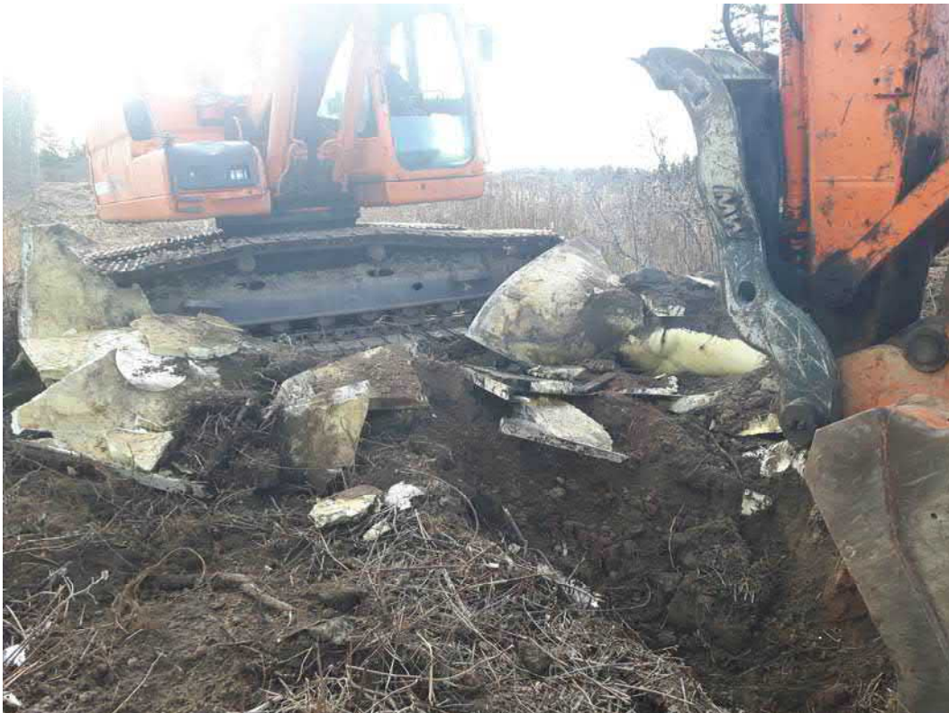
Construction debris at the surface of TP17-05.
