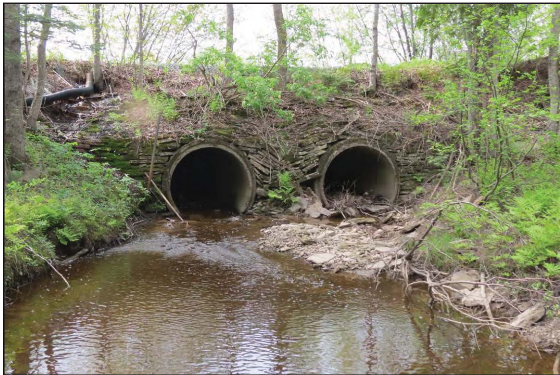
PLATE 2: Concrete and dry stone culvert at Bear Trap Brook in southern end of Section One; facing south; May 30, 2014.
