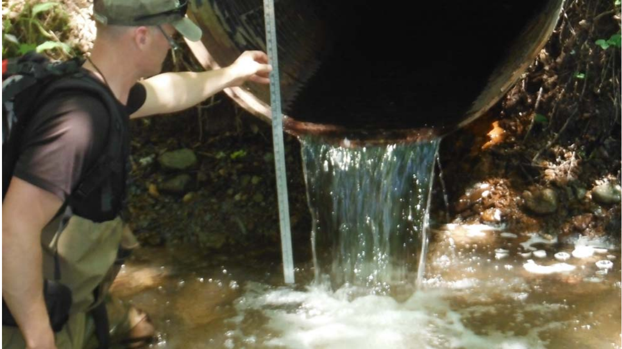
Photo 5: Watercourse 1 – Downstream end of perched culvert under Whitebone Way
