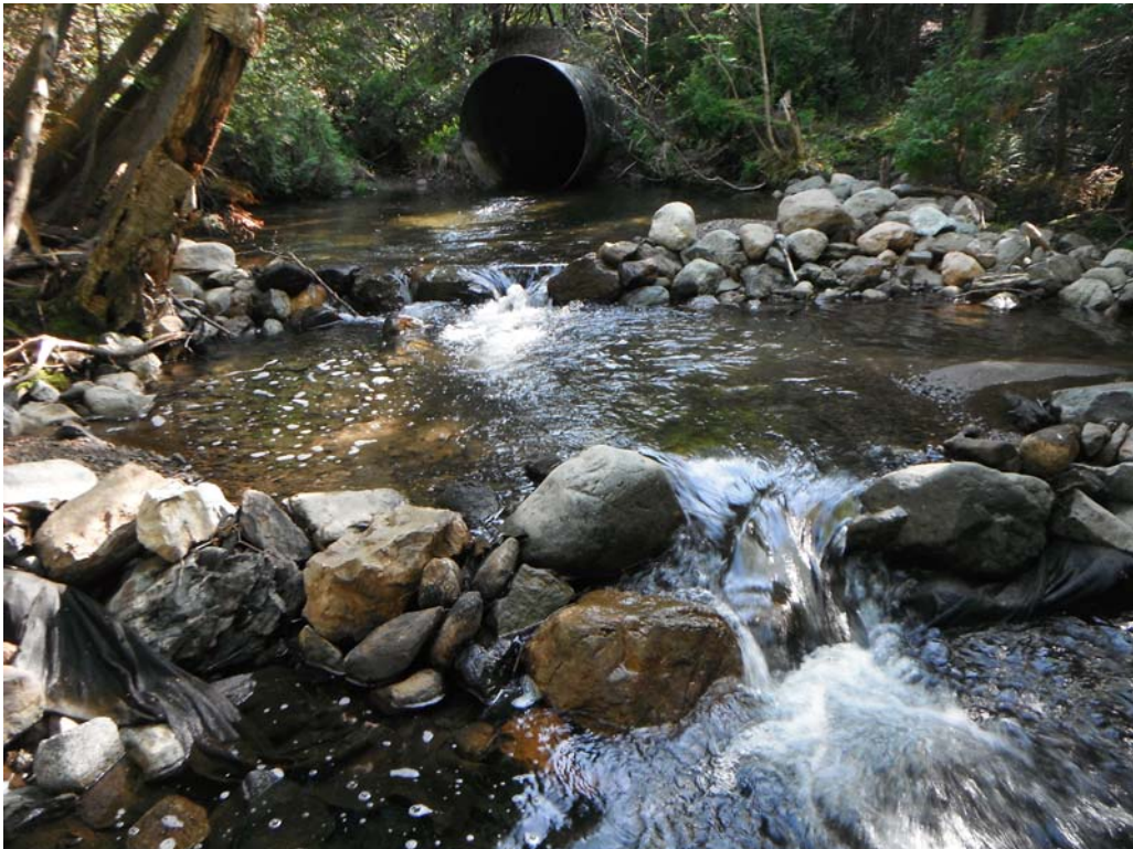
Photo 6: Watercourse 2 – Habitat downstream of culvert under decommissioned rail line and typical of the watercourse
