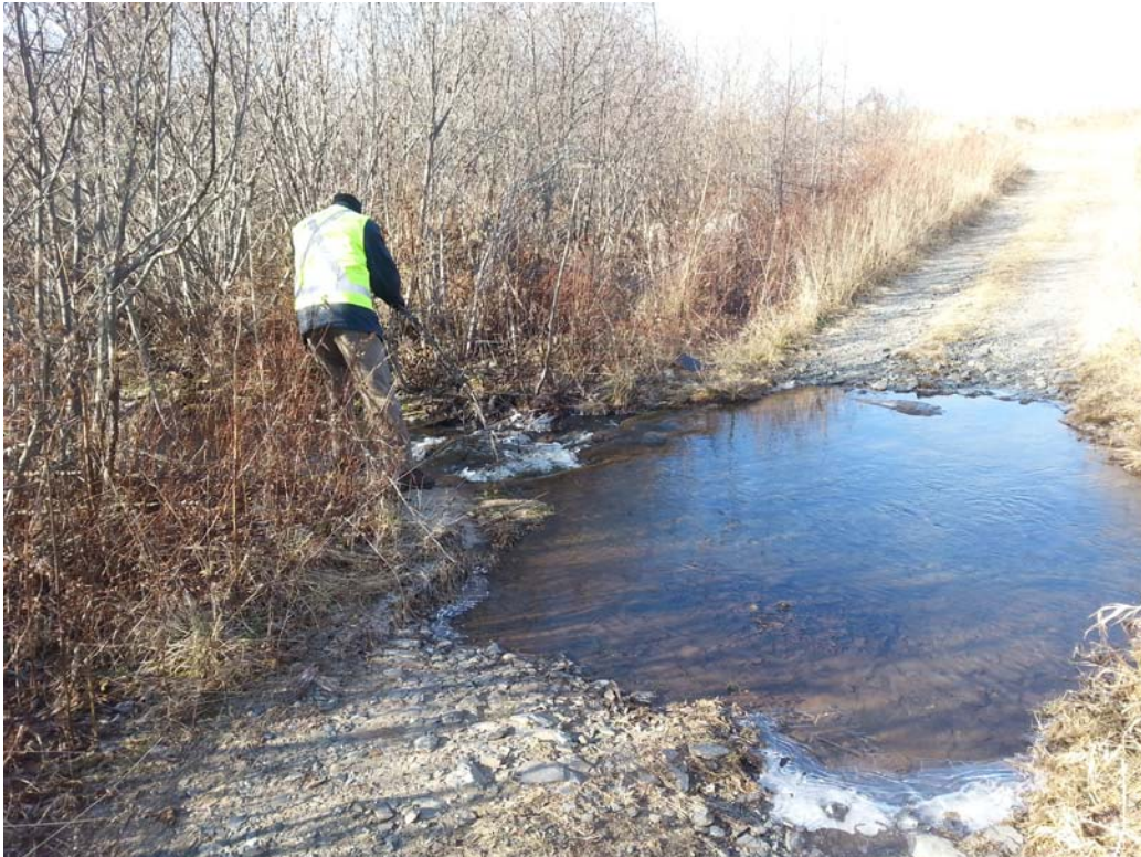
Photo 22: Watercourse 8 – Ponded water on access road (no culvert observed)
