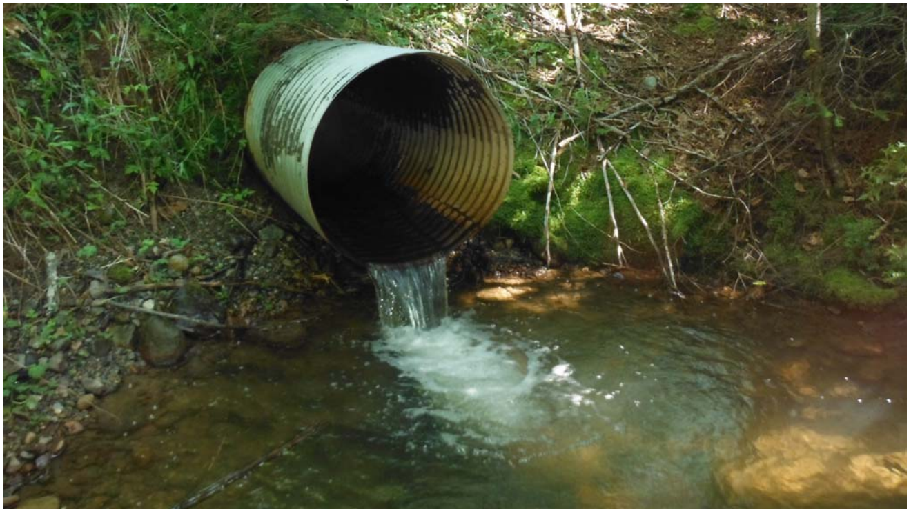
Photo 2: Watercourse 1 – Downstream of perched culvert under decommissioned rail line
